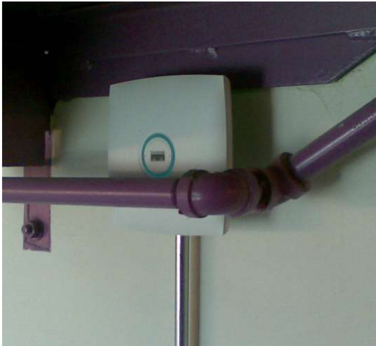
Ceiling mount AP up against pipe
